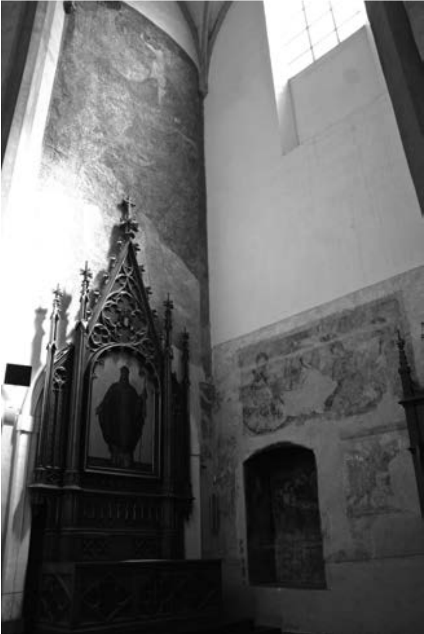
Figure 11.8. Pietà, St George fighting the dragon, the Legend of the Three Living and the Three Dead (the side wall); and St Christopher (the front wall). České Budějovice, Dominican Church of the Presentation of the Virgin Mary, after 1381. Photo: Daniela Rywиковá.
