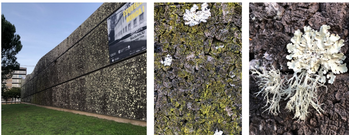
Figure 9. Photographs taken in 2021 of the reconstructed Portugal Pavilion from Expo 2000 in Hannover, in a city park of Coimbra facing the river Mondego after almost 20 years of outdoor exposure. The NE façade is shown (left), as well as details of the uncoated expanded corkboards. Photos by Helena Pereira.
