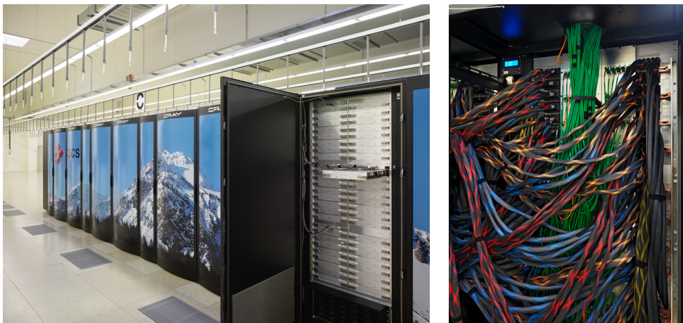
Fig. 37 - 38 Andrea Helbing, Data Center Edges of a Wired Nation , 2018/19
