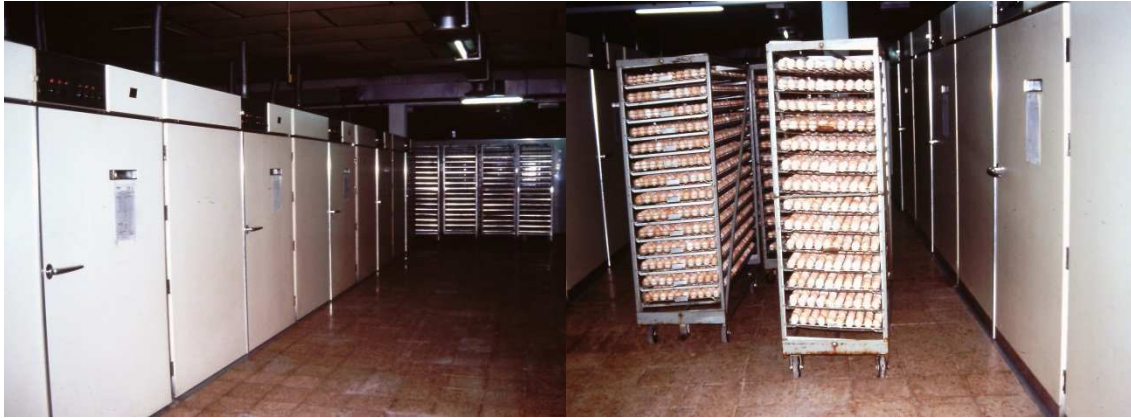
Figure 22. Incubator room and egg trolleys for machine loading (Images graciously provided by DVM Menezes, António).
