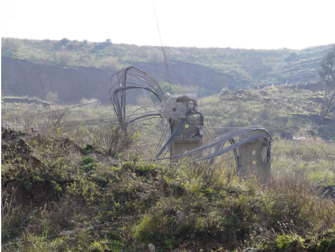
Fig. 0.1 - Damage caused by the landslide on the CREL embankment. Source: Sérgio Cruz de Oliveira, CEG, IGOT, Universidade de Lisboa, 24/01/2010
