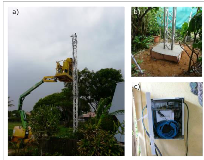
Figure 3.26. Installation of the video monitoring system. a) camera fixing on tower; b) detail of tower base with cement plinth; c) weatherproof box hosting NAS and PSU.
