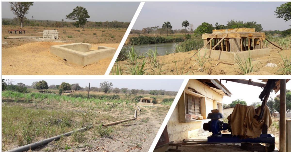
Figure 5:7 The Tede Project: Top(right): Water chamber under construction for the later transferred GYES launching; Top (left): Stand for water storage tank under construction by the waterside; Bottom (right) Power set; Bottom (left) connecting pipes with the stand at the background. Source: Daniel Adayi
