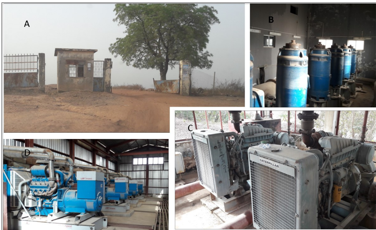
Figure 4:4 Doma Project: (A) Main entrance [south]; (B) & (D) Compressor systems (C) Power Generator. Source: Daniel Adayi.
