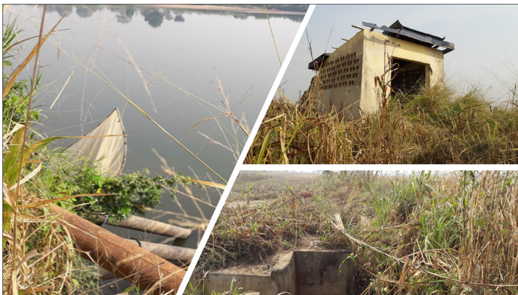
Figure 6:1: Katsina-Ala Project irrigation facilities showing the pump house [January 2017] (top-right); the water suction pipes at the edge of the river (left) and the distribution chamber (bottom-right). Courtesy: Daniel Adayi.
