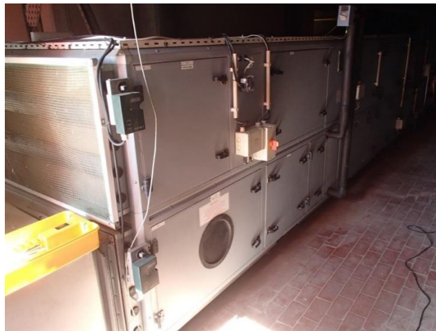
Figura 23: UTA instalada no LNEG
