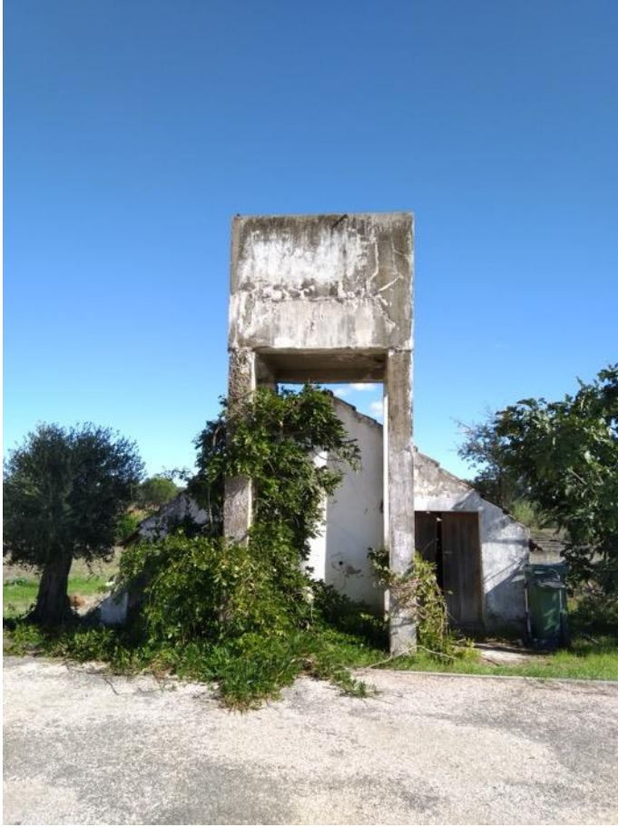
Figure 38. A water tank during September in Grândola, Alentejo, Portugal, 2018. Photo: author.
