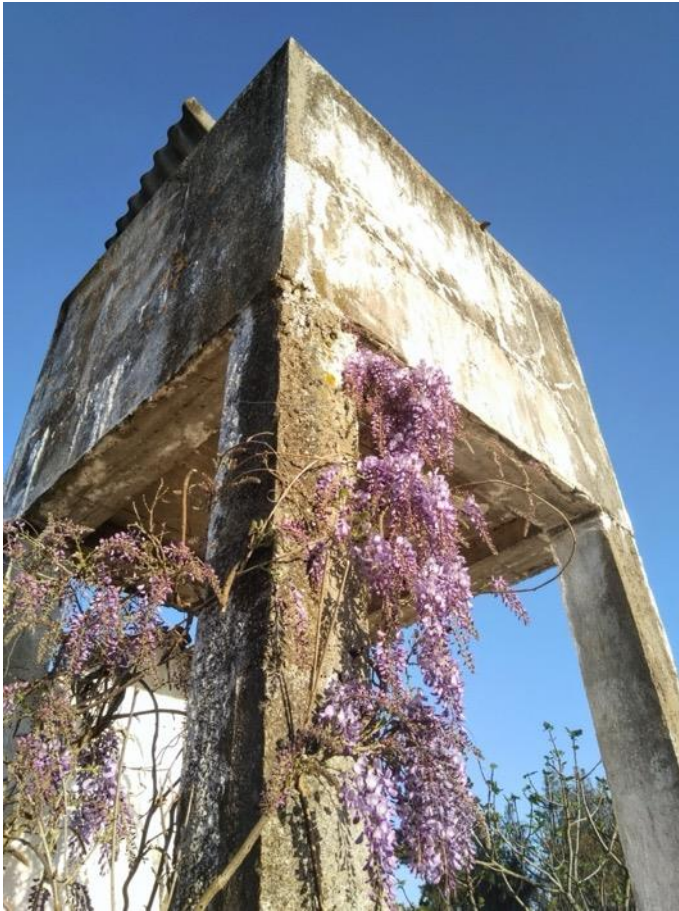
Figure 50. A water tank in Grândola, Alentejo, Portugal, ca. January-April 2019. Photo: author.
