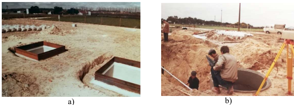
Figure 5. Installation of drainage lysimeters (a, left) before insulation, visible the thin upper wall and, in distance, the bags containing the soil extracted by layers for refilling and (b, right) installation of the pipes bringing the drained water to the wells where water flow would be recorded (1984, Coruche, Portugal).
