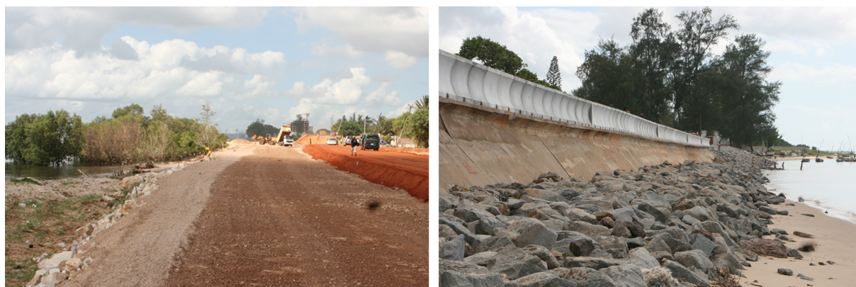
Figure 7. Mangrove destruction for the ring road construction; flood retention wall at Bairro dos Pescadores (2015)
