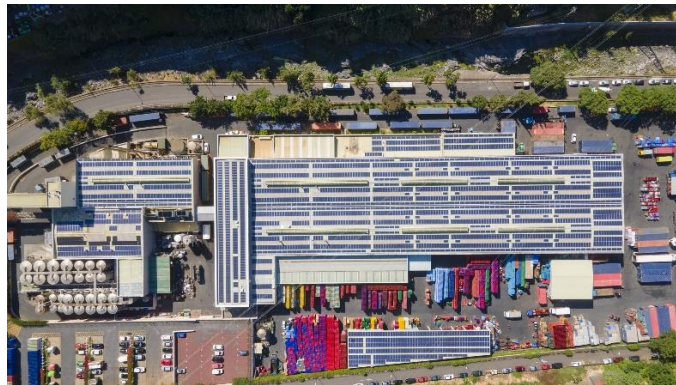
Figure 3 - Photovoltaic panels installed in the roof of ECM's warehouse
