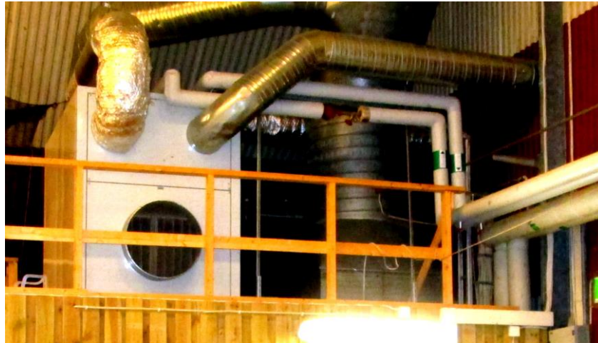
Fig. 5 – Dehumidification system in Nacka ice rink
