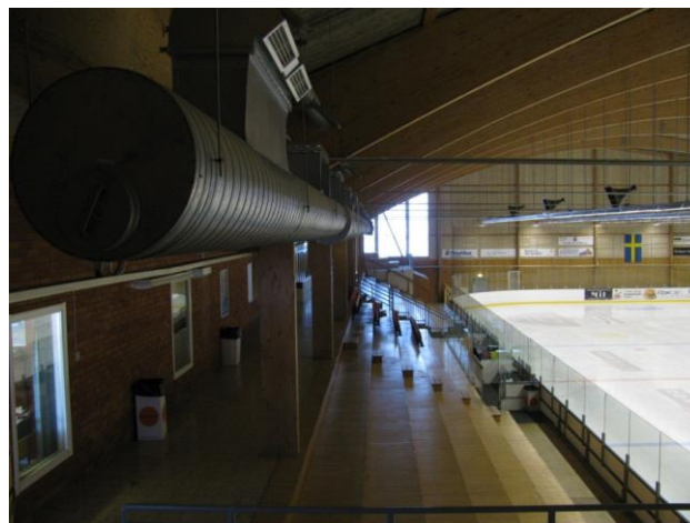
Fig.4 – Ventilation duct over the stands in a Swedish ice rink [3].
