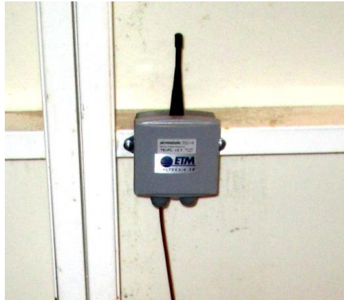
Fig.20 – Example of a sensor responsible to measure temperature and relative humidity
