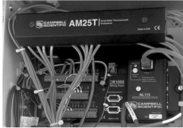
Figure 33 – Multiplexer and datalogger inside the instruments cabinet on the chassis.
