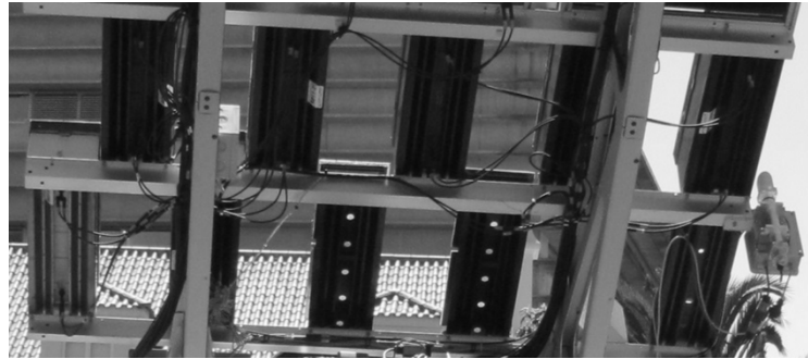
Figure 32 – Back view of the modules on the tracker chassis.
