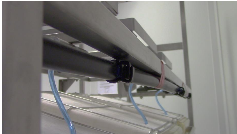
Photo 6. Detail of the water tubs – clamps to seal the system
