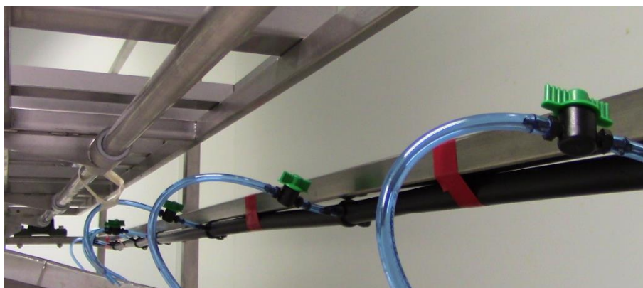
Photo 7. Detail of the water tubs – mini taps to control water volume
