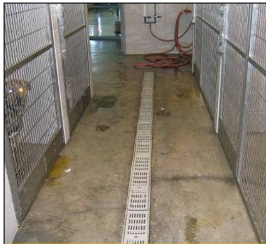
Figure_Apx 1 - Inappropriate drain placement (from Jones, 2007).
