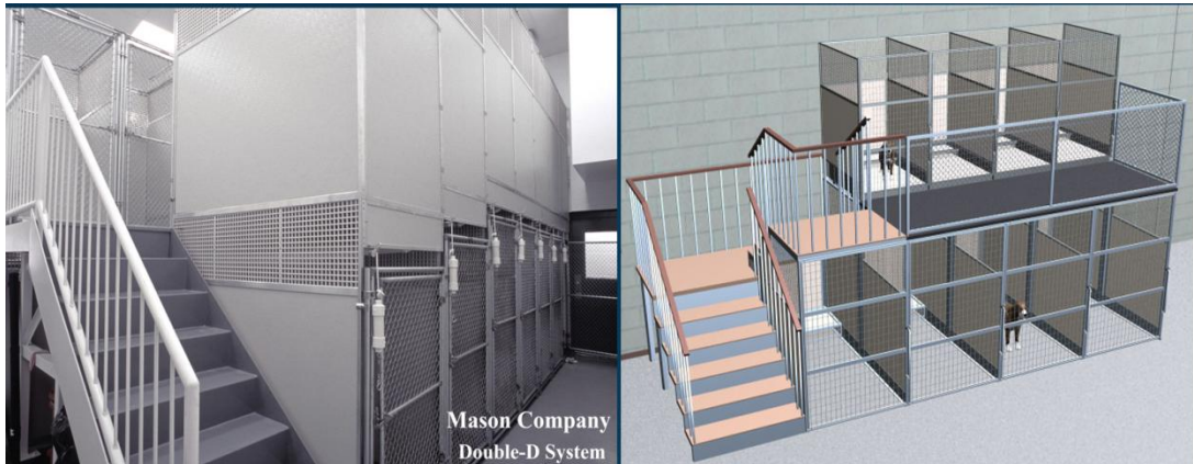
Figure 14 – On the left image a Double-D Kennel System installed at HSP by the Mason Company. On the right, the computer sketch of the kennel. In each suite there was one Double-D System (from www.masonco.com ).
